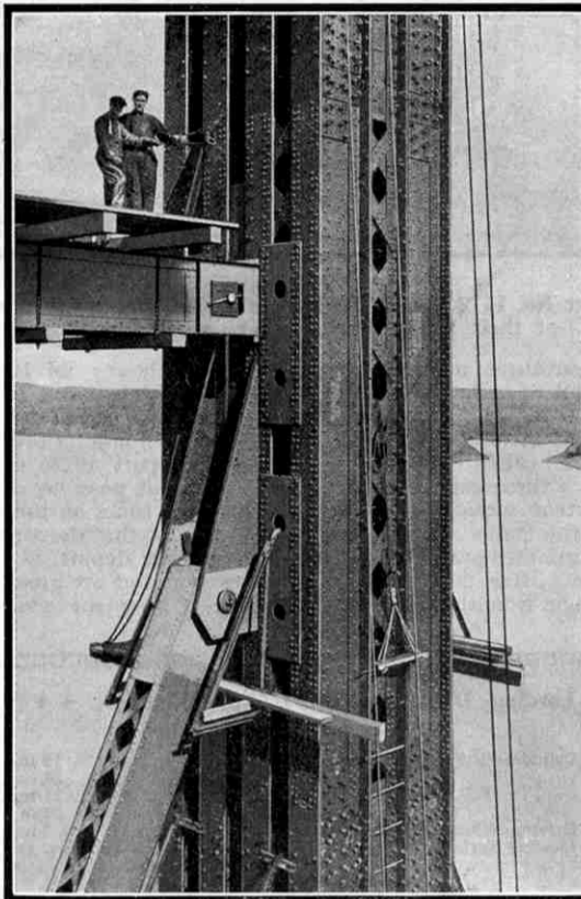
Connecting up one of the web members of the Quebec Bridge. This photograph gives an excellent idea of the immense thickness of the upright girders
