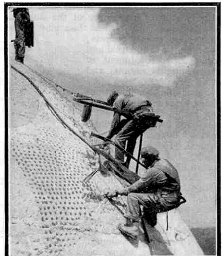
Workman breaking out rock between shallow drill holes being put in by the man at his right.
