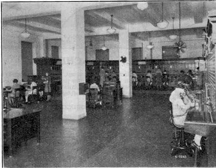
Interior of a large manual operated telephone exchange, showing the extensive switchboard.
