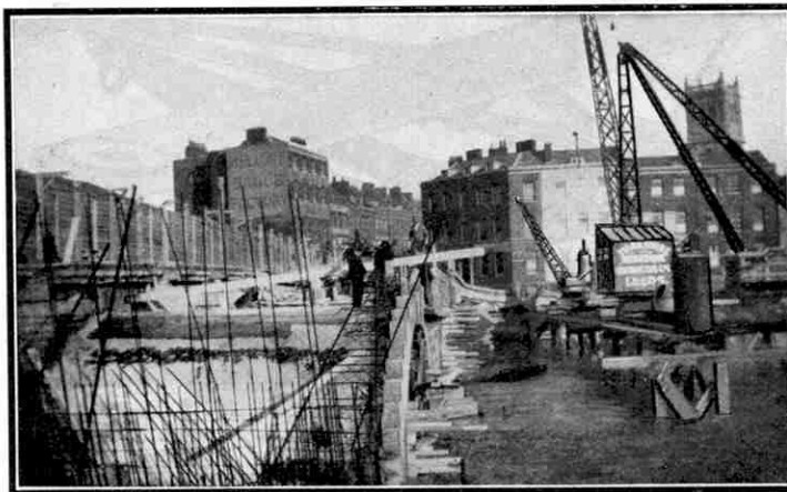
The reconstruction of Worcester Bridge. The steel rods employed to reinforce the concrete are clearly shown in our photograph, taken by our contributor, G. P. Goodall, Worcester.
