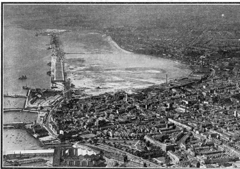
Looking down on the Southampton Dock extension works. On the right of the new quay is the large area of reclaimed land. This and the two following illustrations are by courtesy of the Southern Railway.
