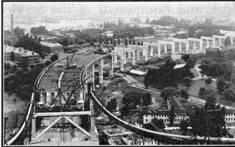
The supporting pillars of part of the viaduct under construction. This view was taken from the top of one of the towers of the East River suspension bridge.
