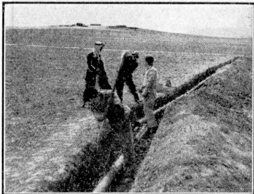
The water pipe line approaching a settlement in the Negev. Arab neighbours took a keen interest in the work.
