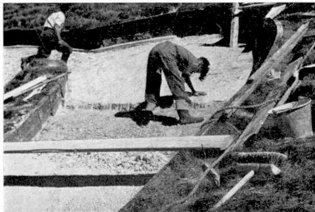
Replacing the tail of the Westbury White Horse by a mixture of cement, chalk and gravel. Photograph by Geoffrey N. Wright, Limpey Stoke.
