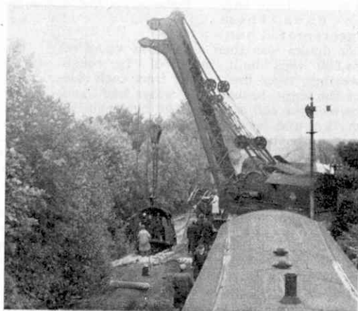
Two 36-ton cranes preparing to lift the engine, as seen from the roof of the breakdown train.
