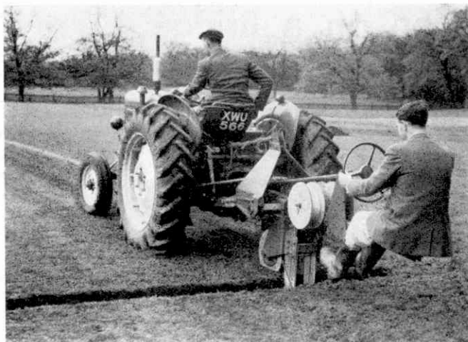
The David Brown Albion underground cable-laying machine at work on a sports ground. Photographs by courtesy of David Brown Tractor Division.
