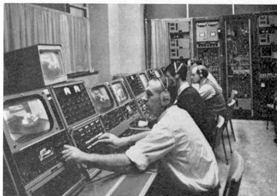
A view of the camera control consoles and equipment racks at English Electric House. Photograph by courtesy of the Marconi Company Ltd.
