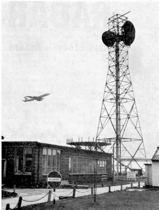
Left, Marconi microwave aerials at Southern Air Traffic Control Centre (near London Airport). The three dishes receive signals from the radar sites at Ash, Ventnor, and Cleve Hill.
